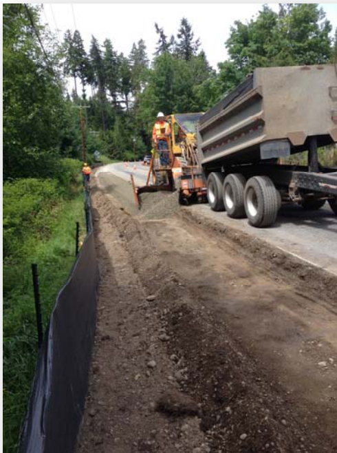
Improvements to this section of Paradise Bay Road include expanding the shoulders to 4' wide, then paving the new surface.
