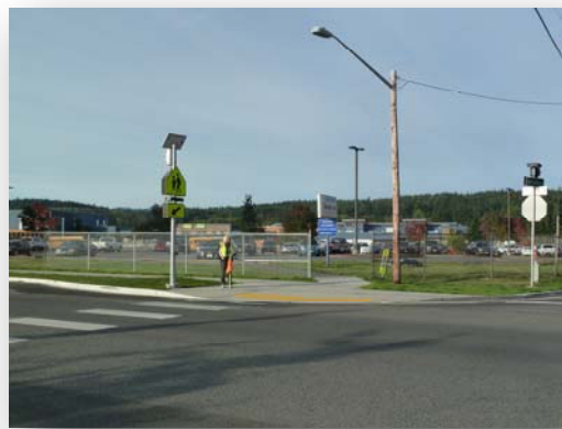
Safe Routes to School improvements included upgrading the crosswalks, installing sidewalks, school zone beacons and additional signage.
